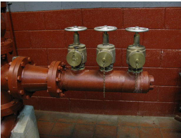
Fire Department Test Manifold
