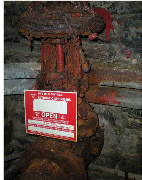
Corroded Curb Valve in Sidewalk Vault
