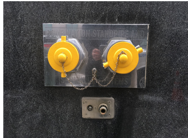
Sprinkler & Standpipe Fire Department Connections
