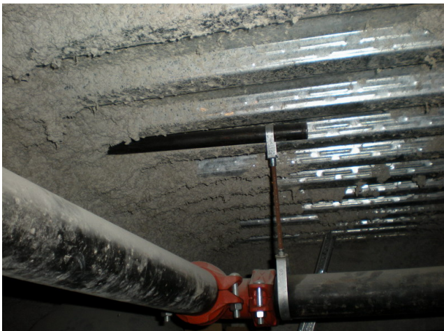
Sprinkler System Improper Hanger
