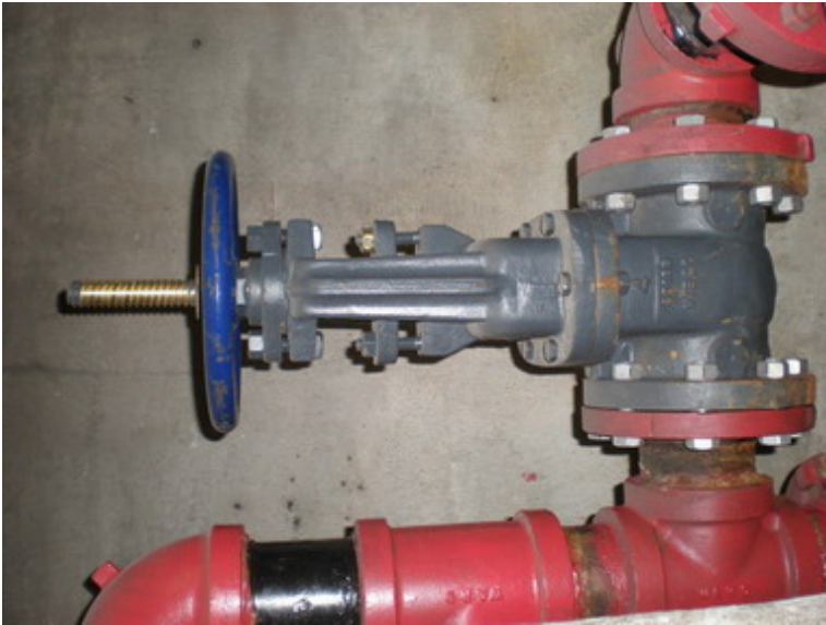
OS & Y valve Not Sealed, Locked, Electronically Monitored, Labeled and Valve Handle Not Painted
