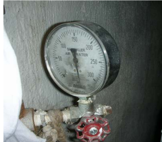
Defective Water Pressure Gauge Exposed to Freezing Temps
