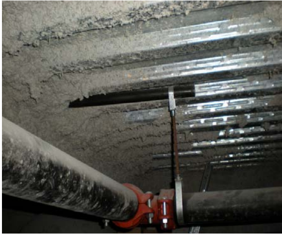
Sprinkler System Improper Hanger
