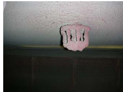
Loaded Sprinkler in Head Guards
