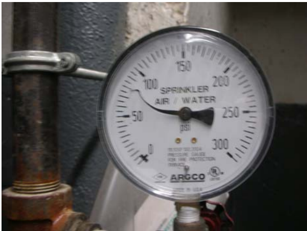
Defective Water Pressure Gauge
