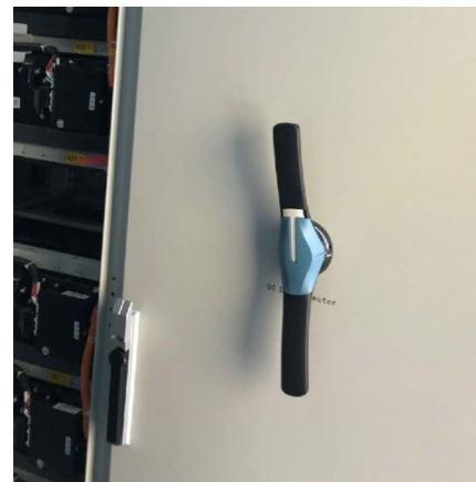
Battery container disconnect switch
