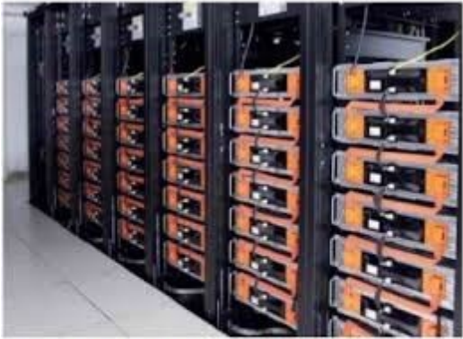
LITHIUM-ION RACK (MULTIPLE MODULES)
