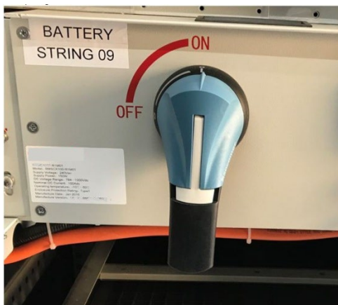
Battery string disconnect switch
