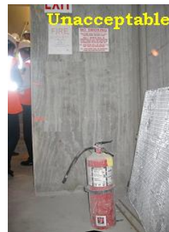
Improper floor placement of Fire Extinguisher.
