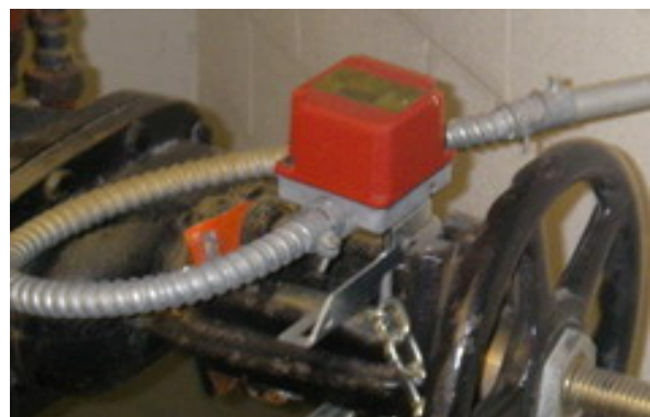
Tamper switch on a sprinkler valve
