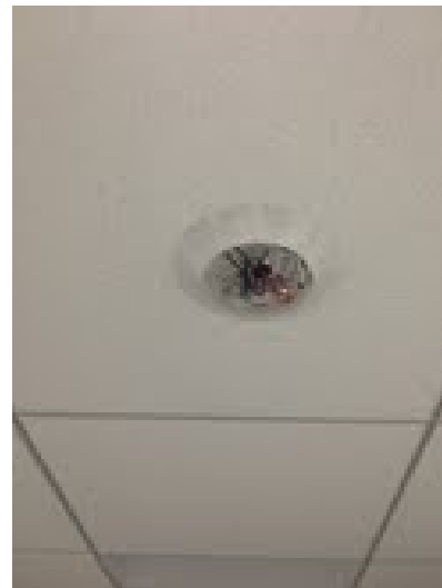
← Detector head missing from its base .
