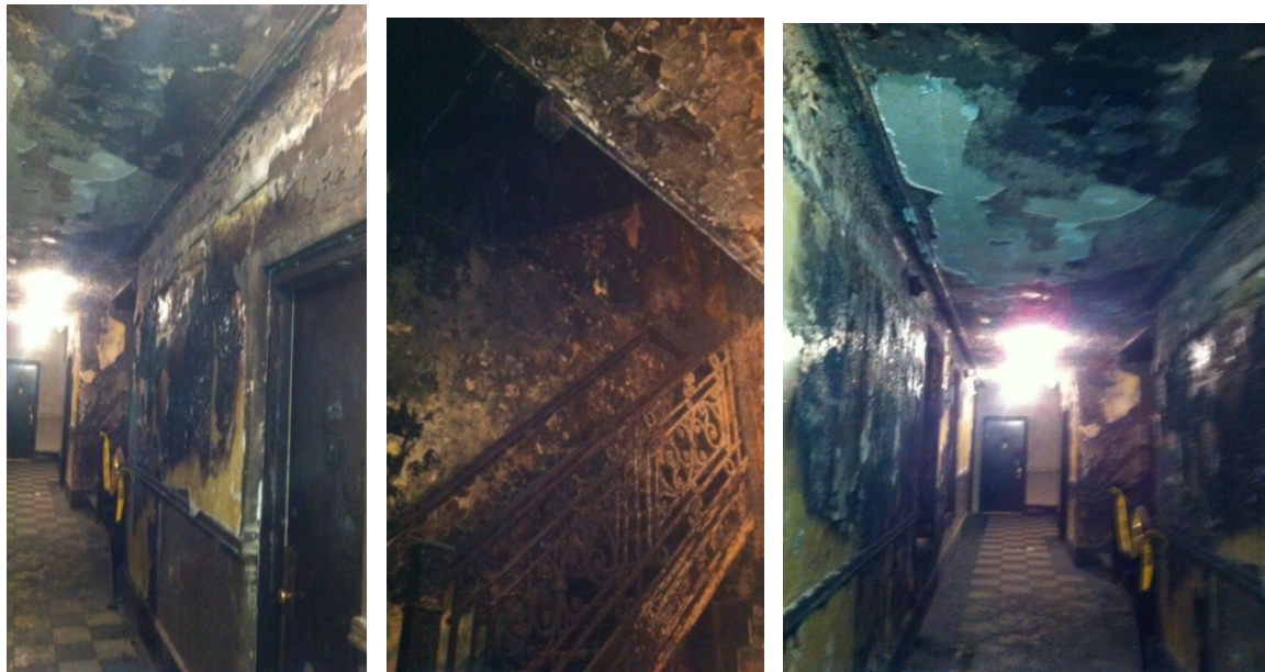
Pictures show the interior of the Bronx, NY shelter after the second mattress fire. There was severe smoke and fire damage in the hallways and stairwells.
