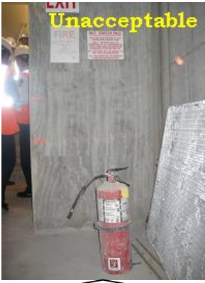
Improper floor placement of Fire Extinguisher.
