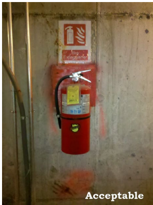
Fire extinguisher in a construction site.
