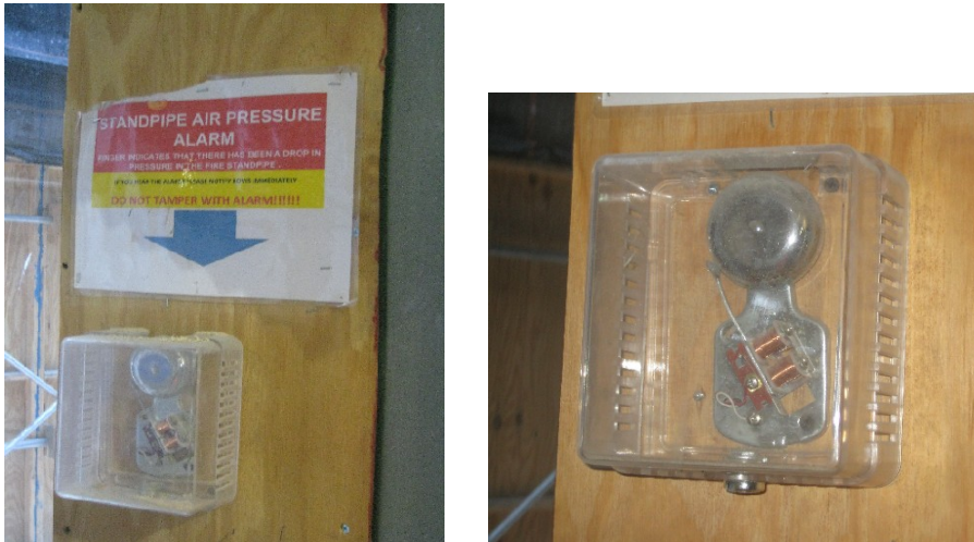
Figure 4-14. Standpipe alarm system
