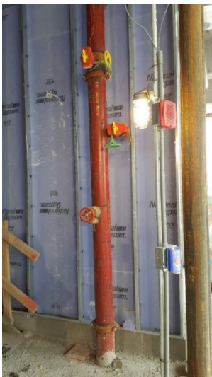
Figure 4-2. Standpipe at Construction Site
