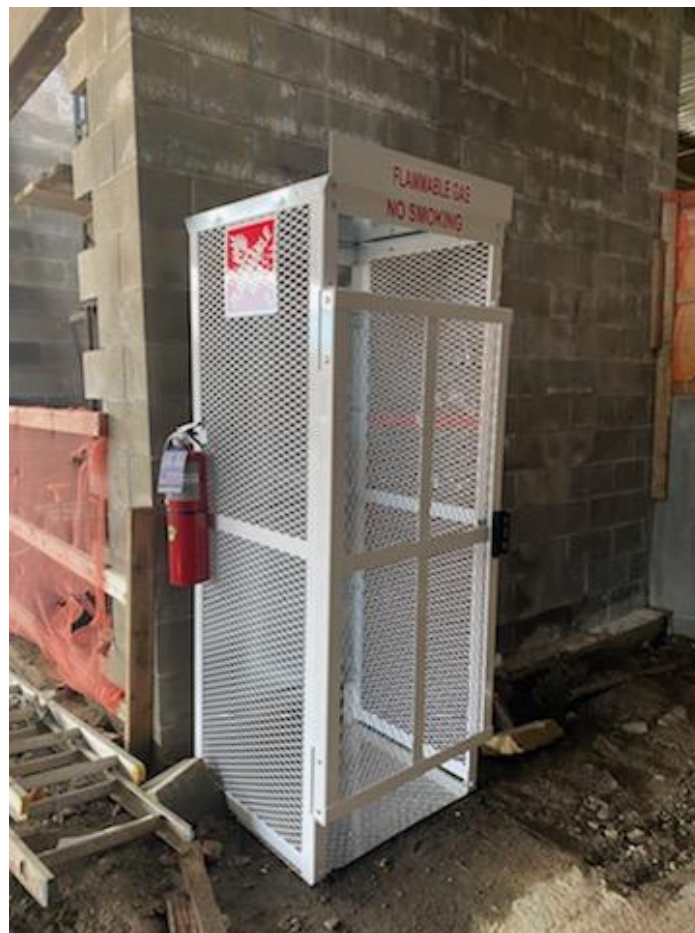
Figure 8-3. Acceptable storage enclosure.
