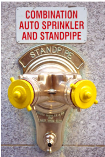
Figure 4-12. The caps of Fire Department connections used for combination standpipe and sprinkler systems shall be painted yellow
