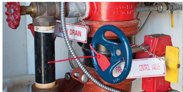
Figure 4-10. This butterfly control valve is locked in open position.
