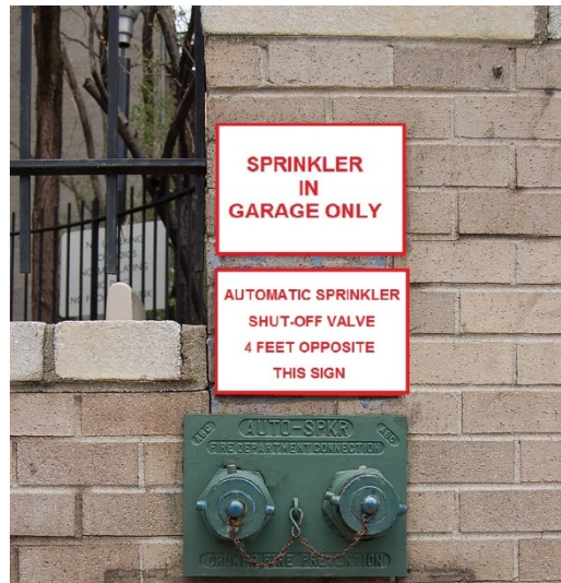
Figure 4-13. Fire Department connections serving a sprinkler system protecting only a portion of a building or structure shall have durable metal signs securely fastened to, or above, the connection indicating the portion of the building or structure protected.
