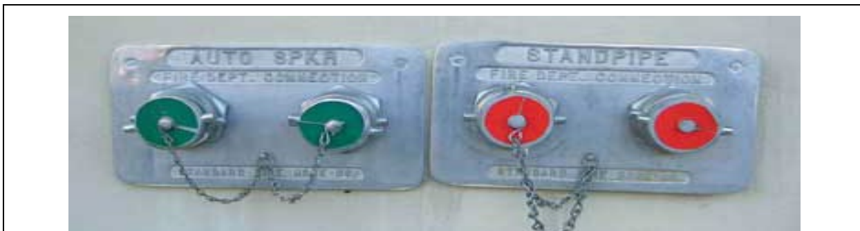
Figure 4-11. Fire Department connections serving a sprinkler system protecting an entire building or structure shall be provided with caps painted green. (left)
